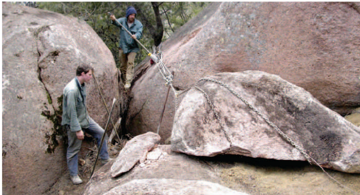
Track workers, Jeram Cowley (left) and Gavin Rose, wrestle a rock into position on a new section of the improved Wineglass Bay track at Freycinet National Park.
